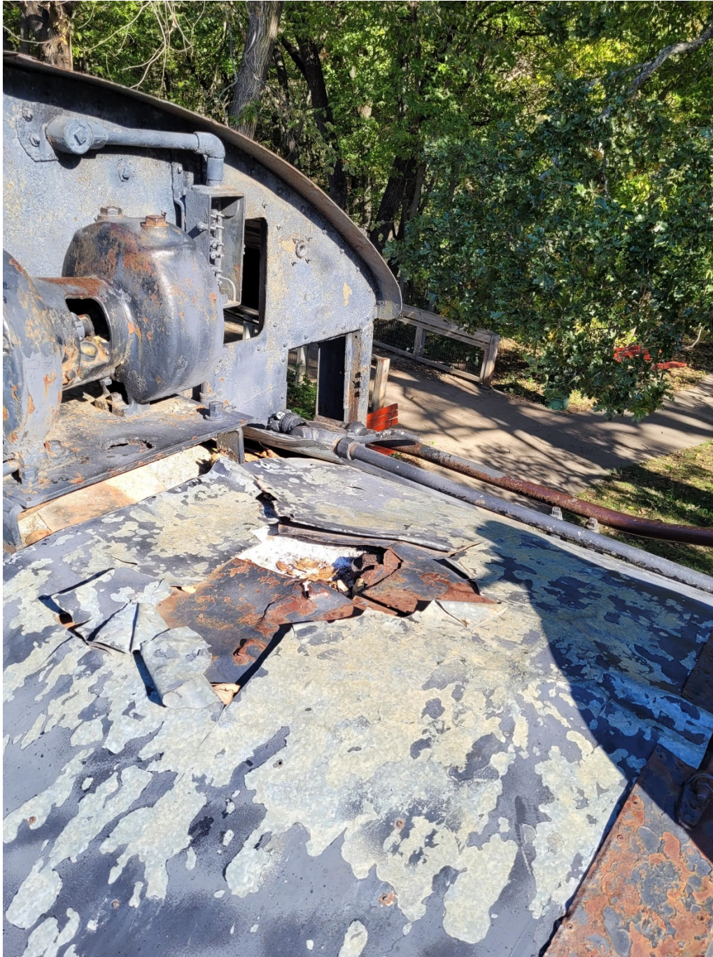
Hole in engine in top of steam drum
