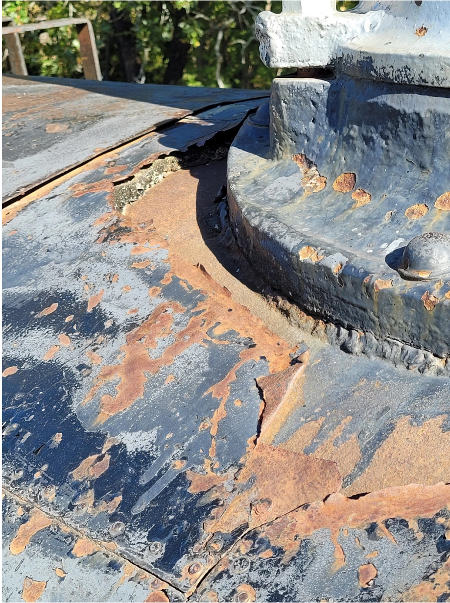
Deteriorated skin on top of steam drum, sharp jagged edges
