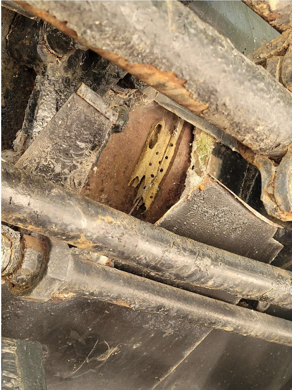
Dislodged cover under steam drum, jagged edges
