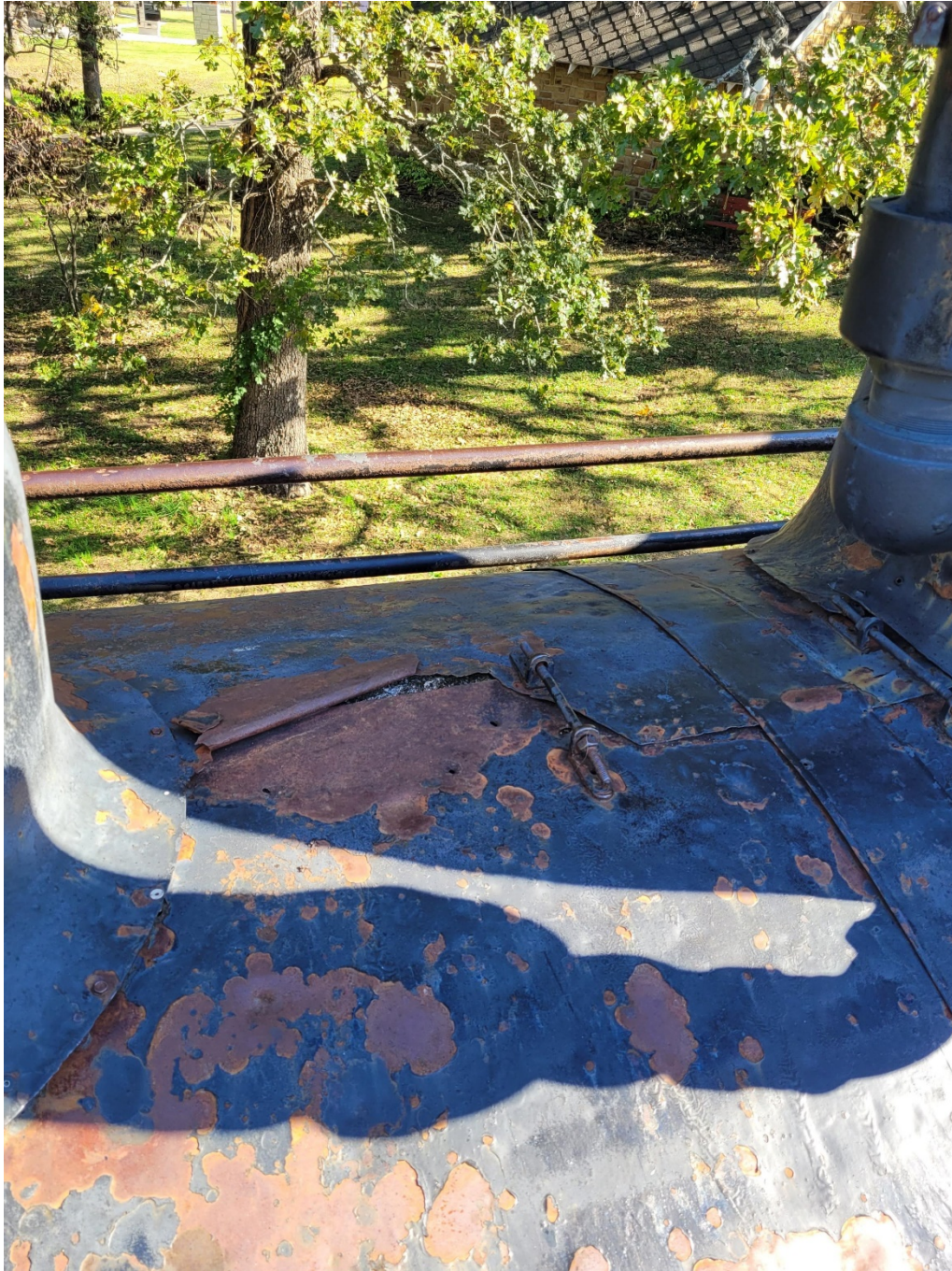
Hole rusted in top of steam drum
