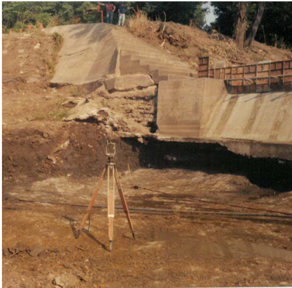
Figure 2. Large void beneath structure (9/12/1988)
