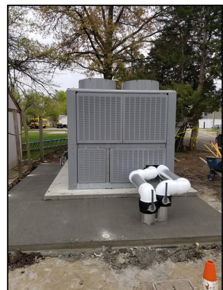
NEW PACKAGED CHILLER AND FOUNDATION
