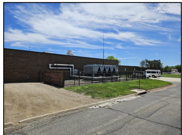
New chiller at Honeybee Lodge – KNI, Topeka, Kansas
