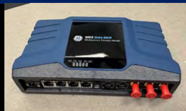
Installed new cellular radios on the airport and college towers, as well as the 17th St. pump station. Installed cellular radios on the north tower and Laurel St. tower
