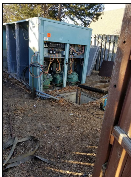
EXISTING CHILLER CONDENSING UNIT
