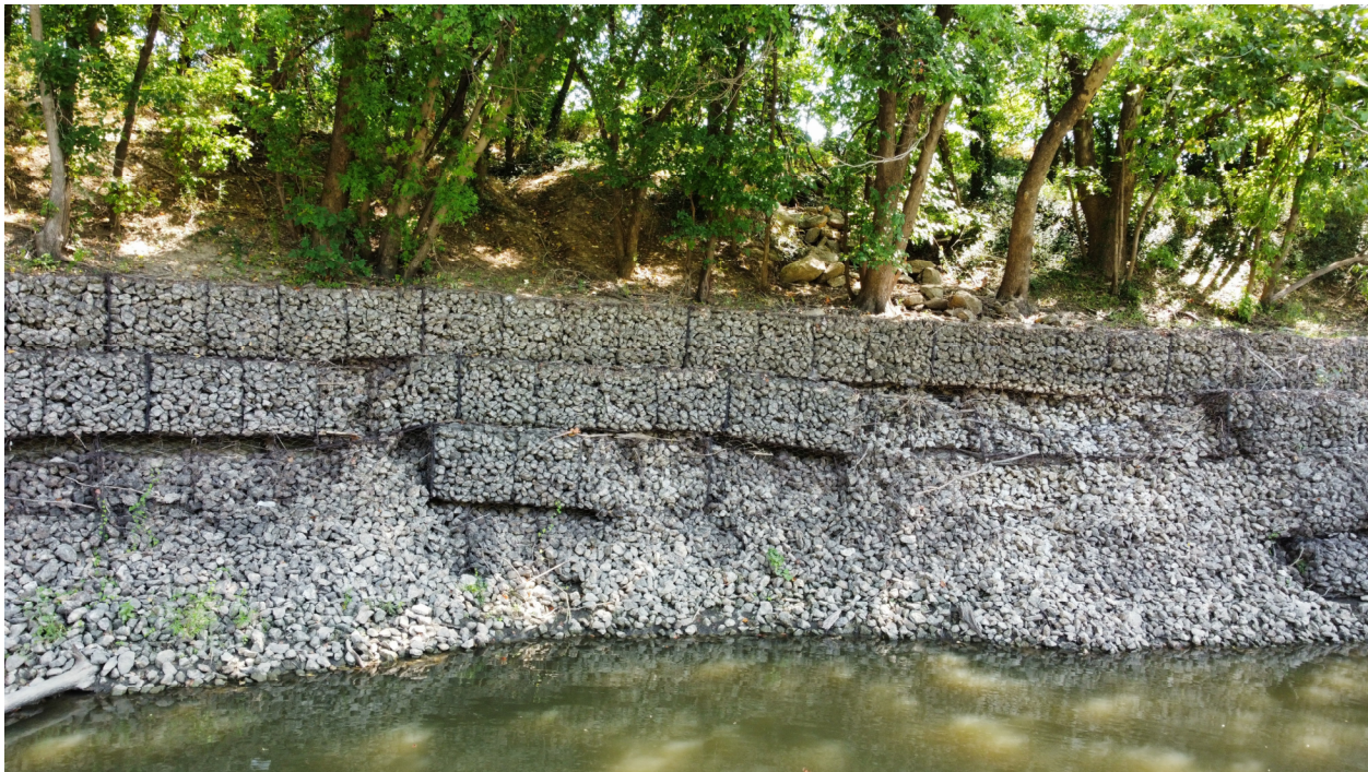
FIGURE 11 - GABION FAILURES ALONG THE DOWSTREAM EAST BANK
