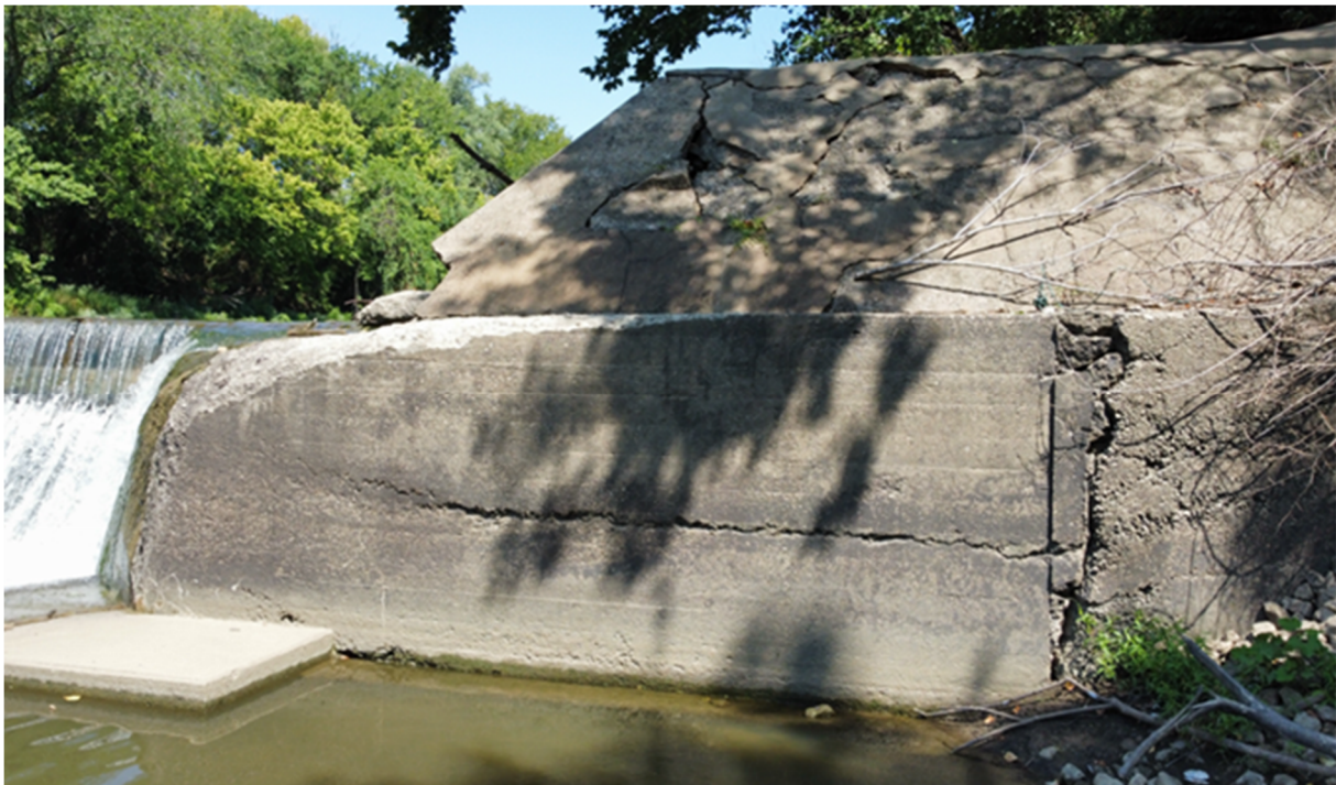
FIGURE 16 - EROSION AND WEATHERING ALONG SURFICIAL CRACKING
