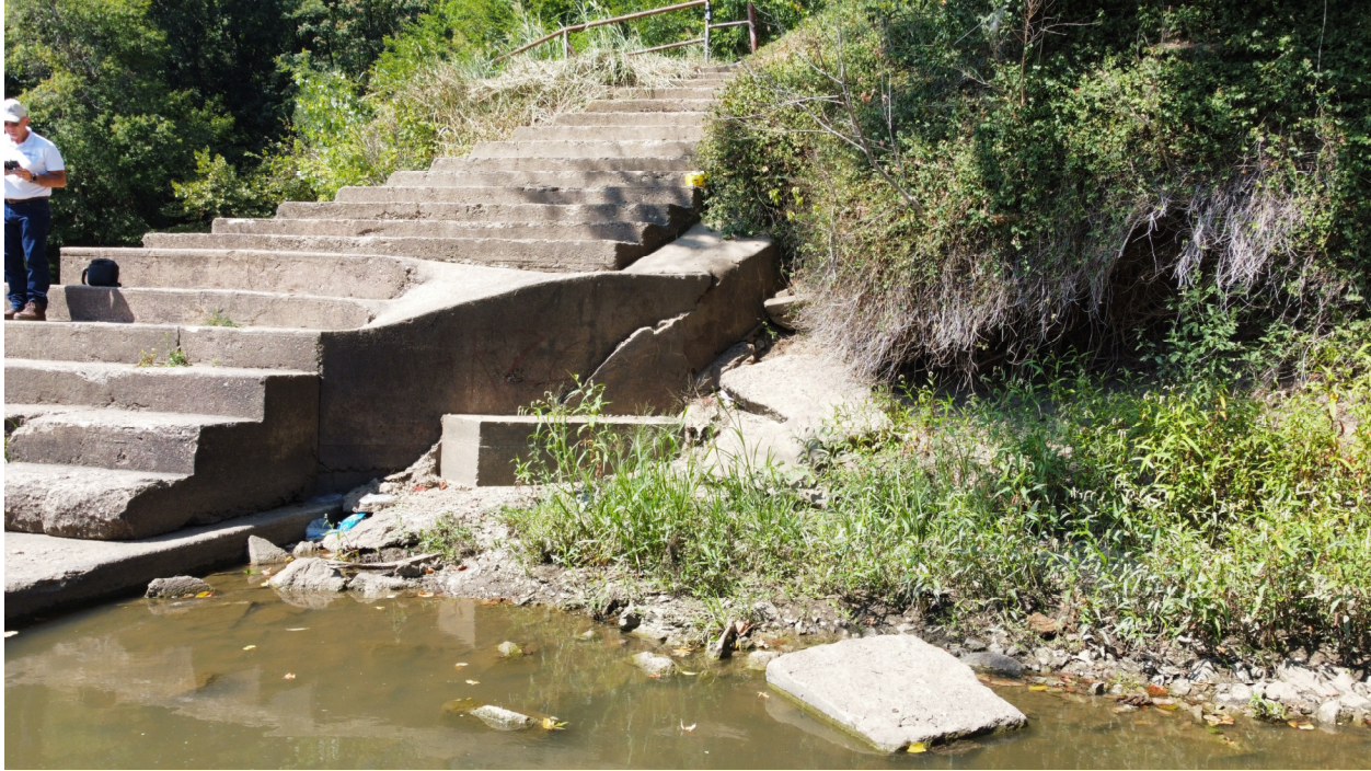
FIGURE 12 - MISSING RIPRAP AND EROSION ALONG THE UPSTREAM WEST BANK
