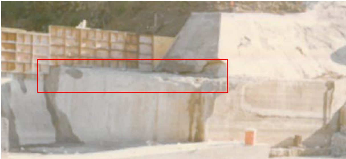
FIGURE 14 - CONSTRUCTION PHOTO SHOWING CONTROL SECTION PRIOR TO DAMAGE, 1988
