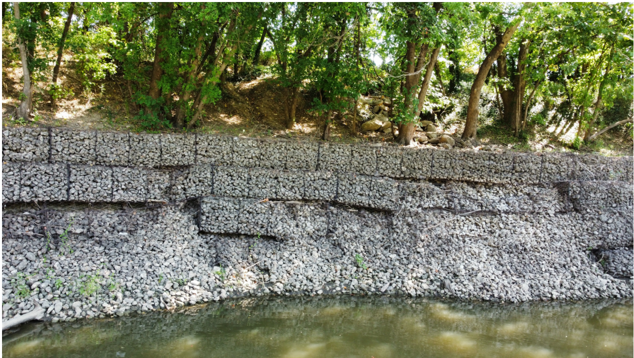
FIGURE 11 - GABION FAILURES ALONG THE DOWSTREAM EAST BANK
