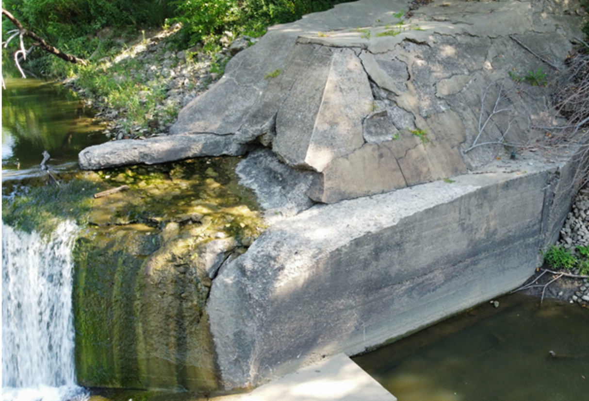
FIGURE 15 - STRUCTURAL DETERIORATION OF EAST ABUTMENT
