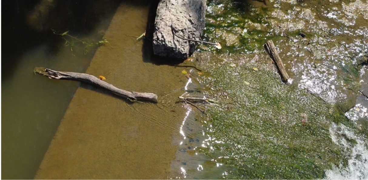
FIGURE 13 - BLOWOUT AND DISPLACEMENT OF CONTROL SECTION, NEAR EAST ABUTMENT
