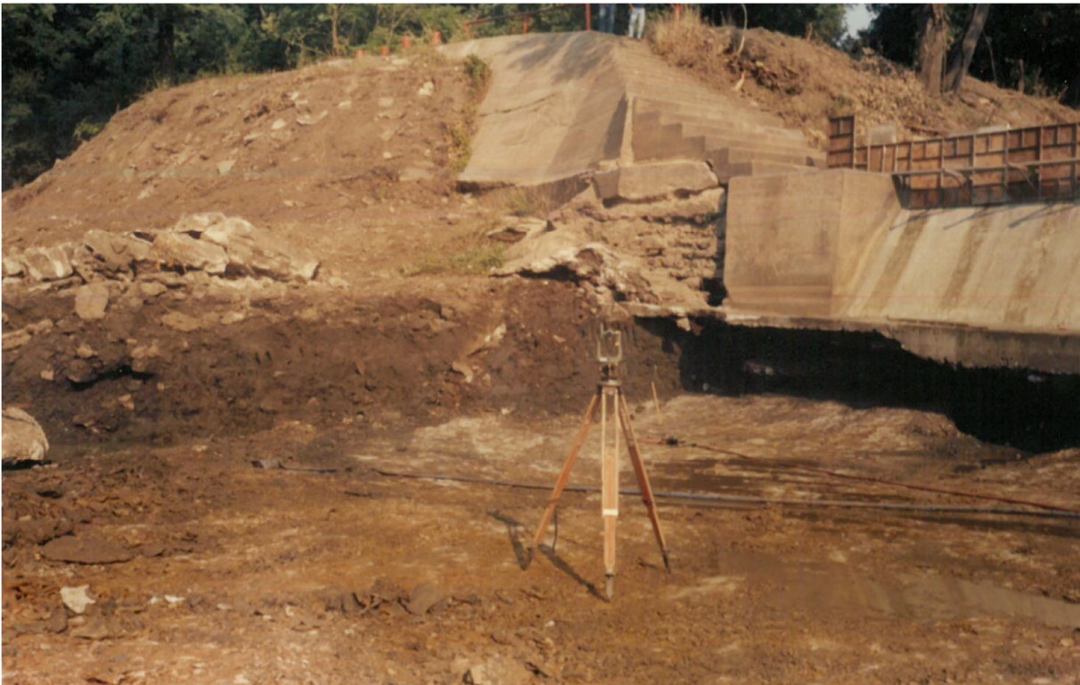
FIGURE 6 - SCOUR HOLE REVEALED UNDER WEST ABBUTMENT/APRON, SEPTEMBER 12, 1988
