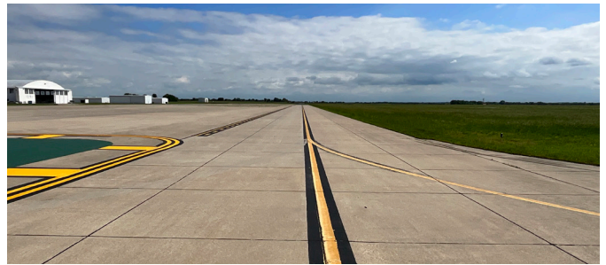
Figure 7: Parallel Taxiway A Pavement Condition
